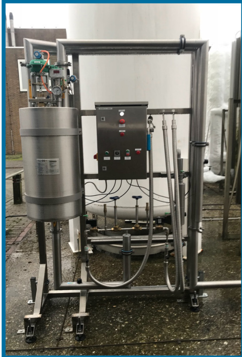
Filling station with uninsulated valves
